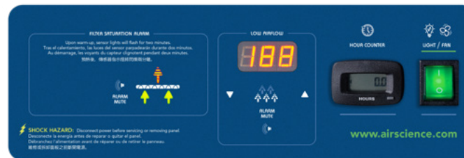
FSA/Autocal Control Panel
